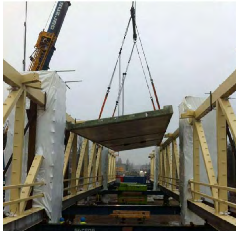
Bridge in Utrecht Infracore technology
